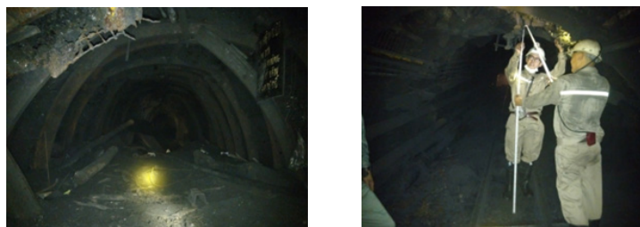
Fig. 7. The collapses of TVT tunnel seam 14.5 southeast area at Khe Cham III coal mine in Quang Ninh coal mine area at 12/05/2021 [1]
