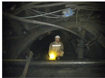
Fig. 5. The collapses of deep underground tunnel floor seam 14.5 southeast area at Khe Cham III coal mine in Quang Ninh coal mine area at 12/05/2021 [1]
