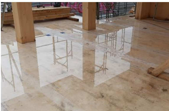
Fig. 6. Water accumulation on undrained floor
