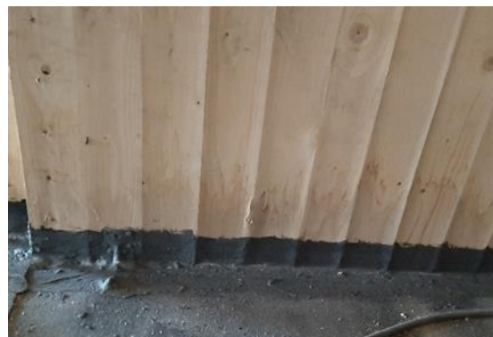
Fig. 7. CLT element after extensive exposure to water
