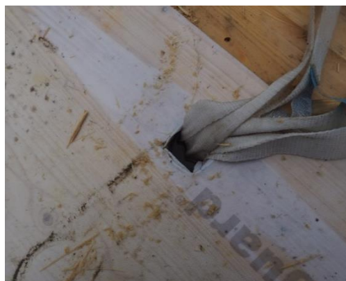
Figure 3. Blind holes pose a risk for the moistening of CLT elements
