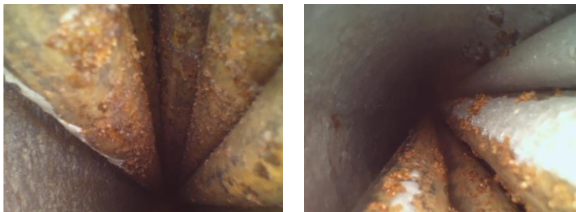
Fig. 11. Tendon ducts without grouting, surface corrosion – corrosion grade 3
