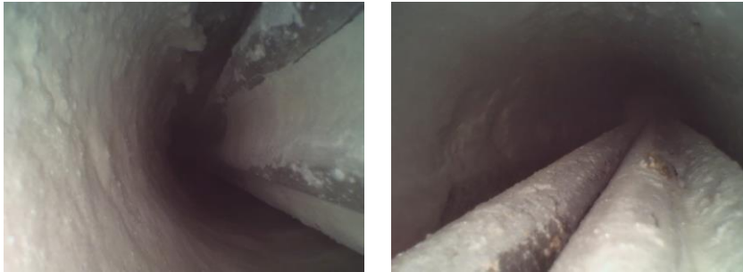
Fig. 9. Tendon ducts without grouting, tendons without corrosion – corrosion grade 1
