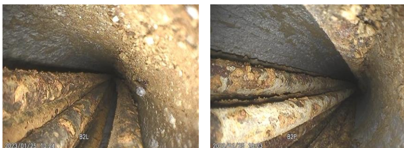
Fig. 12. Tendon ducts without grouting, surface corrosion – corrosion grade 5
