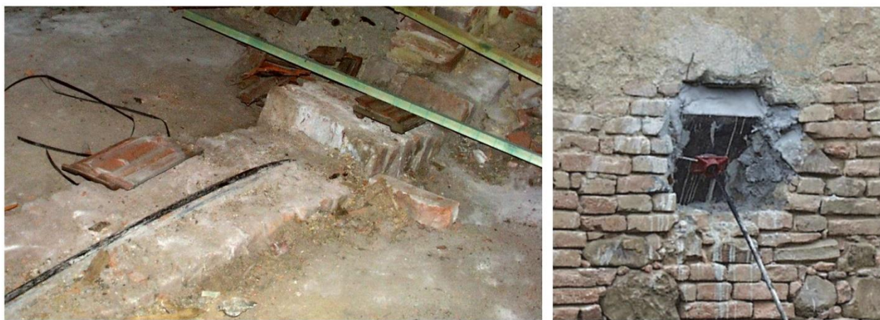
Fig. 3. Leading of the strand above the arch (left) and anchor with the spreading plate (right)
